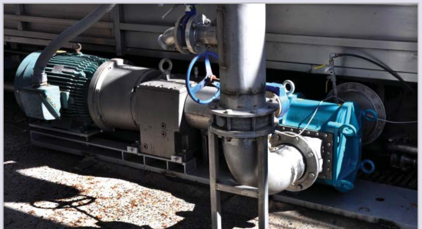
One of the Börger EL-1550 rotary lobe pumps in the MUST processing facility
