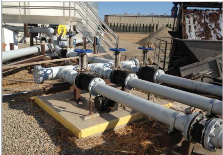
The winery production waste water treatment system
