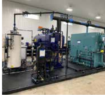
CB Steam Boiler Skid for Campus Commissary
