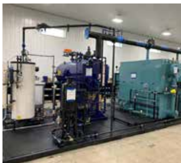
CB Steam Boiler Skid for Campus Commissary
