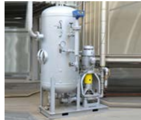
STEAM CONDENSATE RETURN PACKAGE
