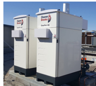
CB Hot Water Boilers for Sacramento Facility
