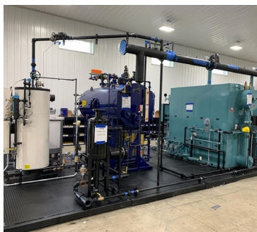
CB Steam Boiler Skid for Campus Commissary
