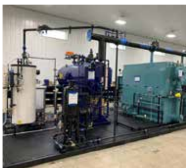
CB Steam Boiler Skid for Campus Commissary
