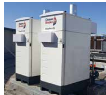
CB Hot Water Boilers for Sacramento Facility
