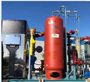
Camus Hot Water Boiler Skid for Commercial Property
