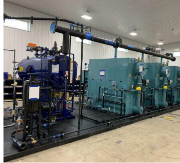
CB Steam Boiler Skid for Campus Commissary
