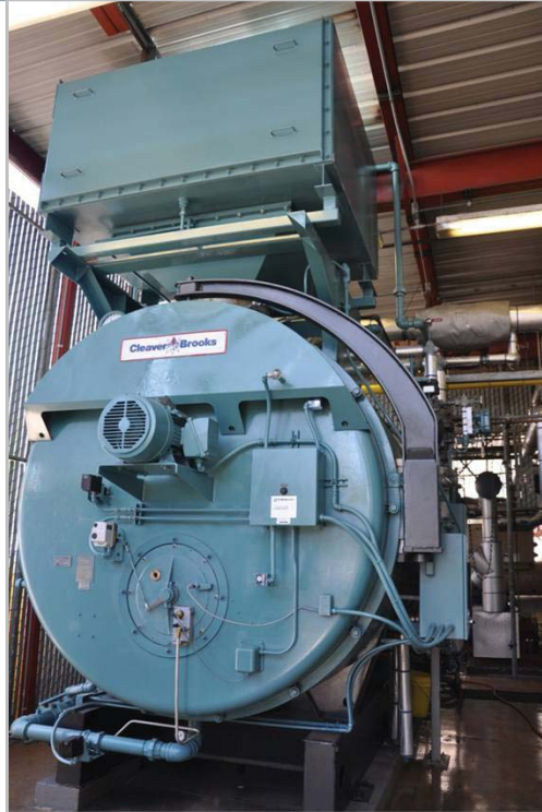
Finished installation of Hawk ICS panel, entrance panel, VFD, ULN burner, and economizer
