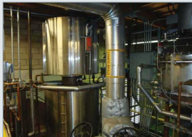
Economizers on mezzanine level
