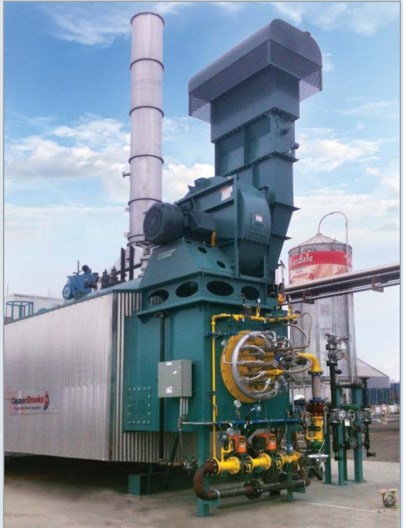
Final installation of the SCR based steam plant fully designed, integrated and installed by R.F. MacDonald Co.
