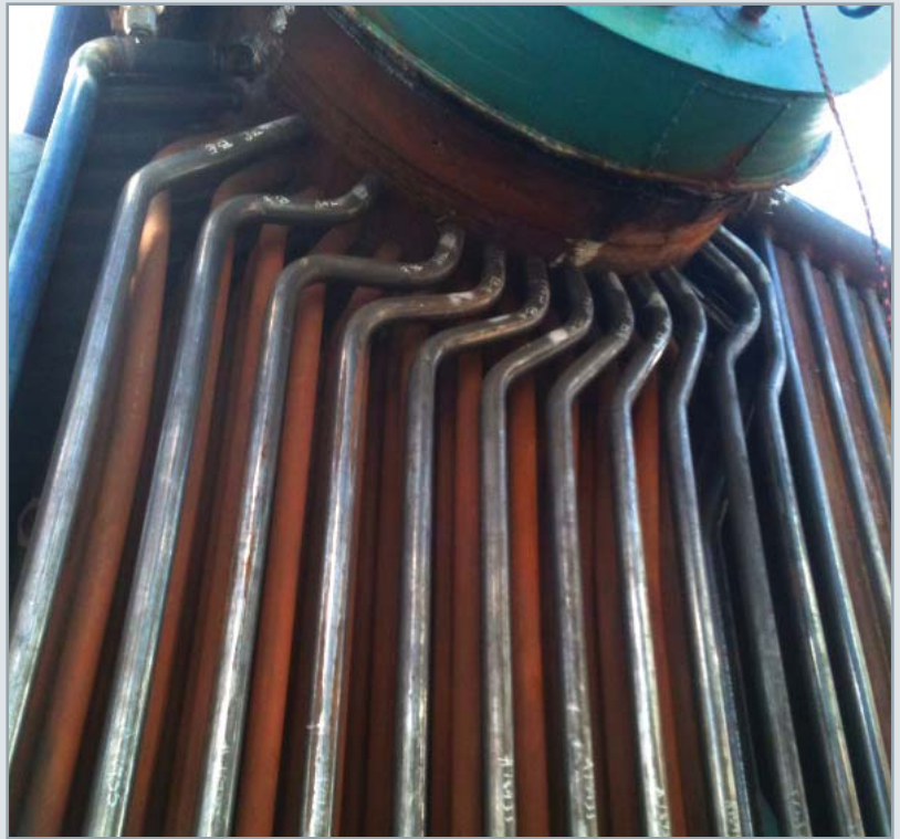
New outside tube sections moulded, welded and installed in the existing boiler
