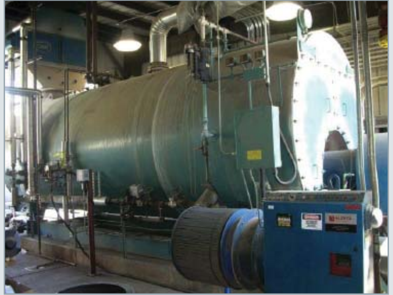
Final installation at the Hilmar Cheese plant
