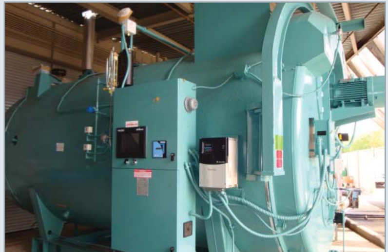
The boiler with the control system in the new installation
