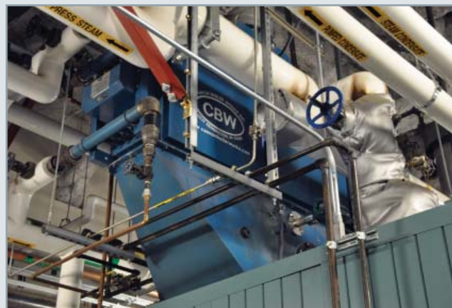
The installation of the feedwater heater helps conserve energy
