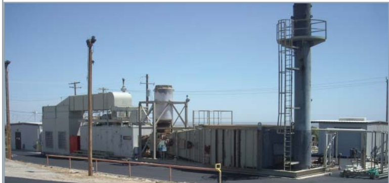
Cogeneration facility with upgraded SCR final installation
