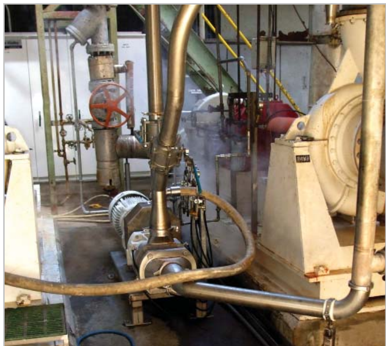
The Bornemann SLH-180 pump installed in the processing plant
