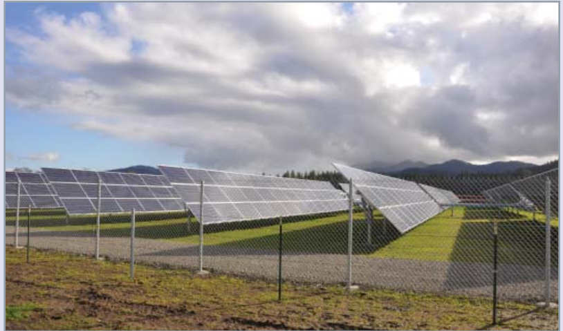
The solar panel fields that supply power to the pumping station
