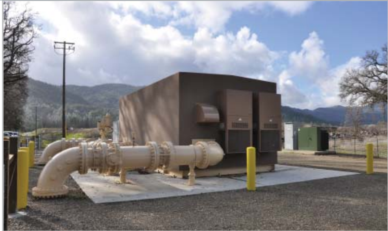
The new Bear Canyon Zero pumping station that boosts pressure in the 50 mile pipeline
