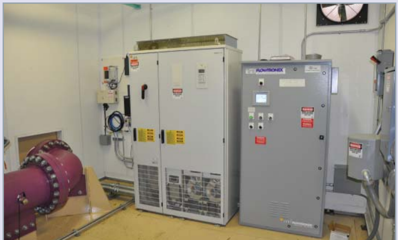
Allen Bradley PLC, ITT PumpSmart and Flowtronix control systems
