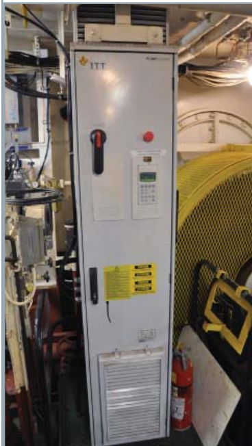
The PumpSmart System Locker
