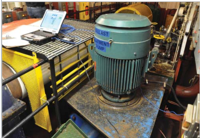
The ballast treatment pump motor, with the majority of the vertically mounted pump beneath the metal divider
