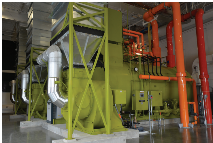
Hot Water Generator
