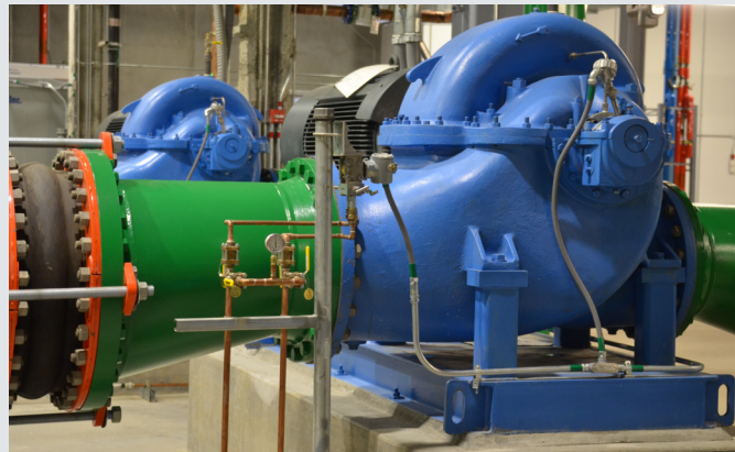
Example of one of the twenty six Goulds pumps installed
