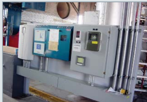
Burner control system with RFM O2 trim and variable speed drive
