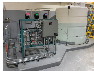
SCR with Non-Hazardous Urea
